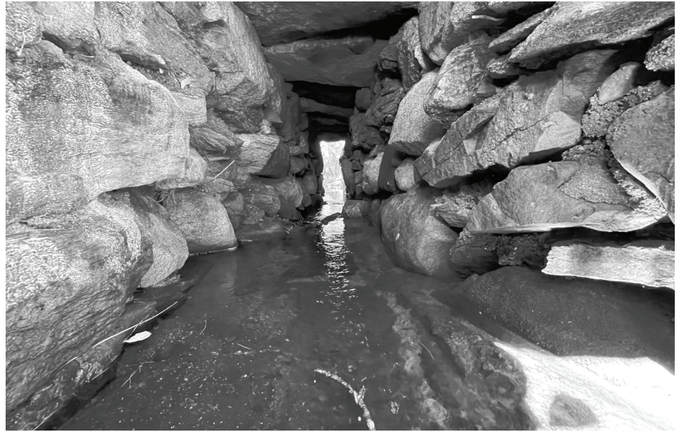
The view inside the stone box culvert located under Middle Road in Tuftonboro. Note the granite slabs resting on stone walls, called "post and lintel" construction.
